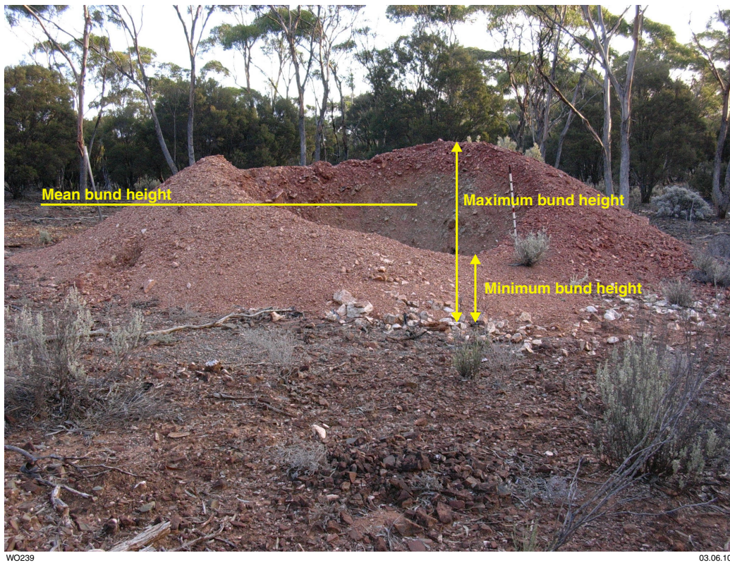
Figure 1.9 A shaft surrounded by a full bund of waste rock showing maximum, minimum, and calculated mean bund heights.
