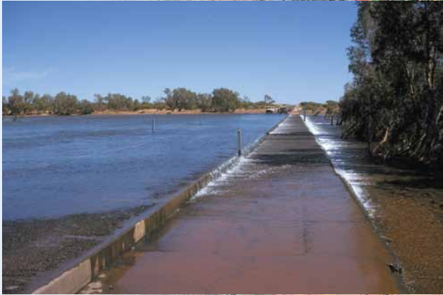
Flooding of the Shaw River, at a concrete causeway where the road and the river meet
